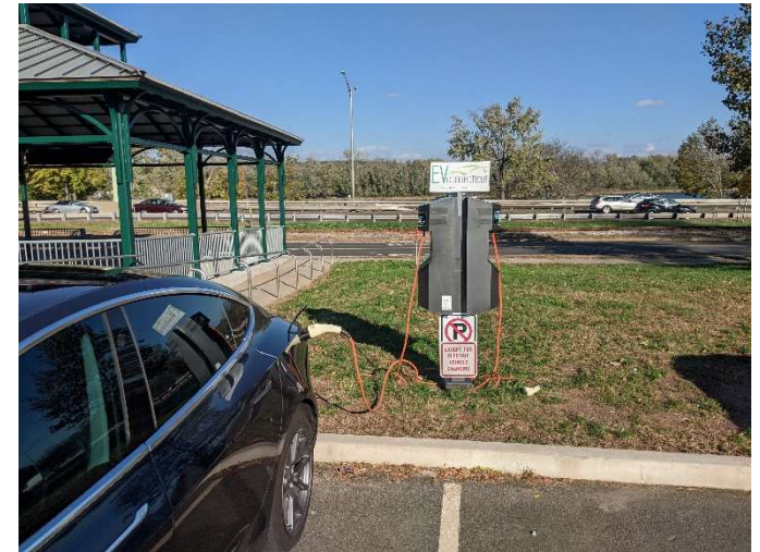
EV Charging Station at City Hall
