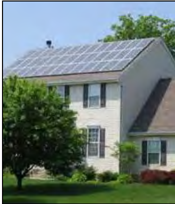
Residential Solar Installation
