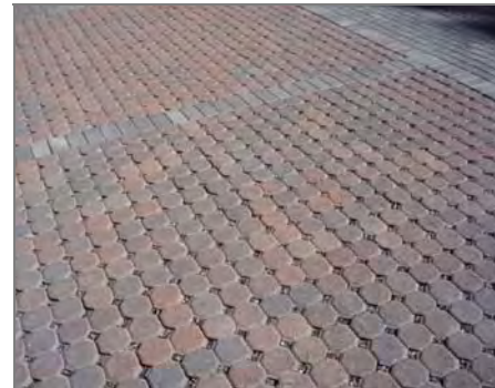
Pervious pavement that allows water to infiltrate soil.
