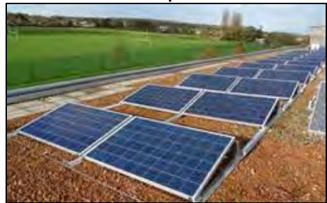
Commercial Rooftop Solar Installation
