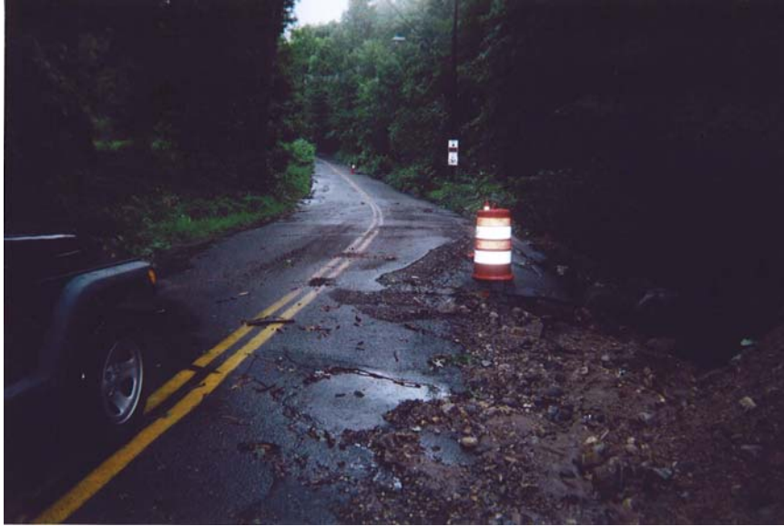
20. Damaged section of East Mountain Road
