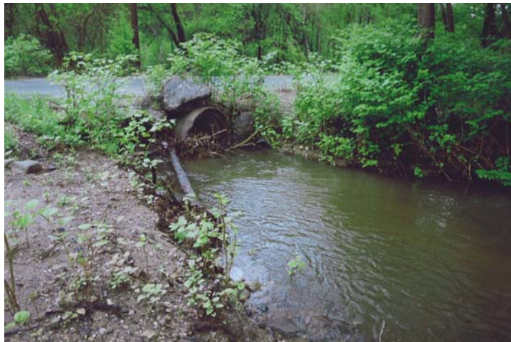
Old Tannery Brook at Nutmeg Valley Street (note blocked culvert)
