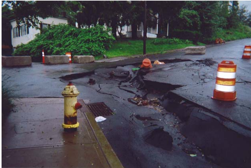
9. Damage to 5 th Street & Bank Street
