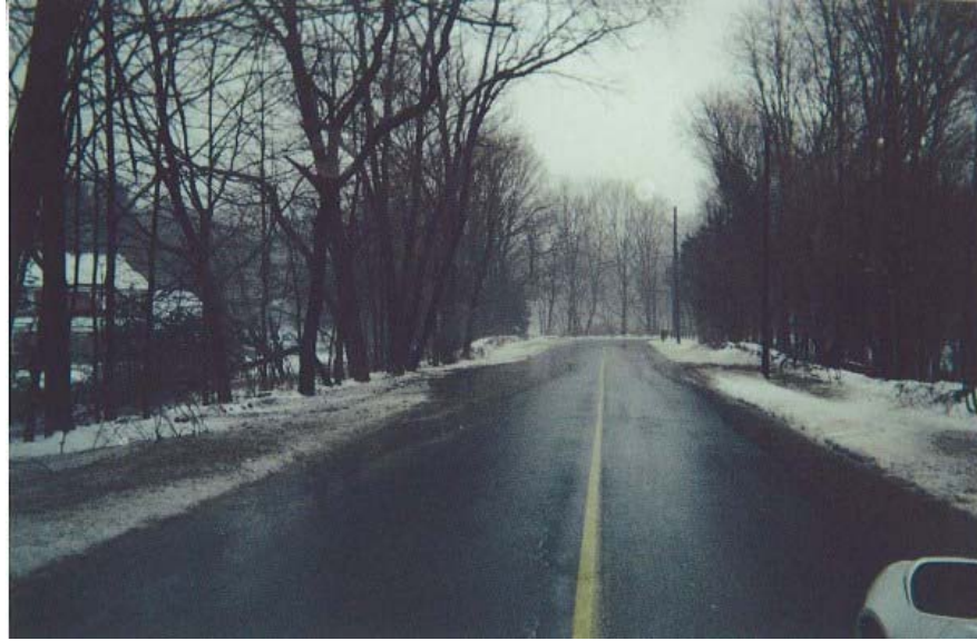
11. Nuisance flooding along Jeremy Swamp Road
