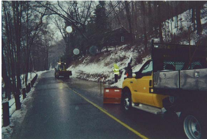
3. The Town of Southbury alleviating nuisance flooding along River Road
