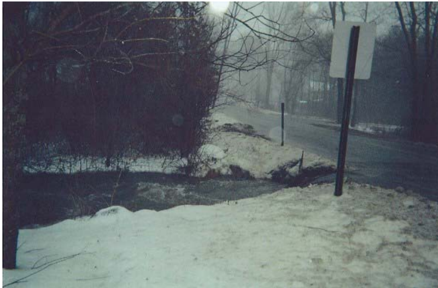
13. View looking south of Jeremy Brook culver crossing outlet along Hulls Hill Road
