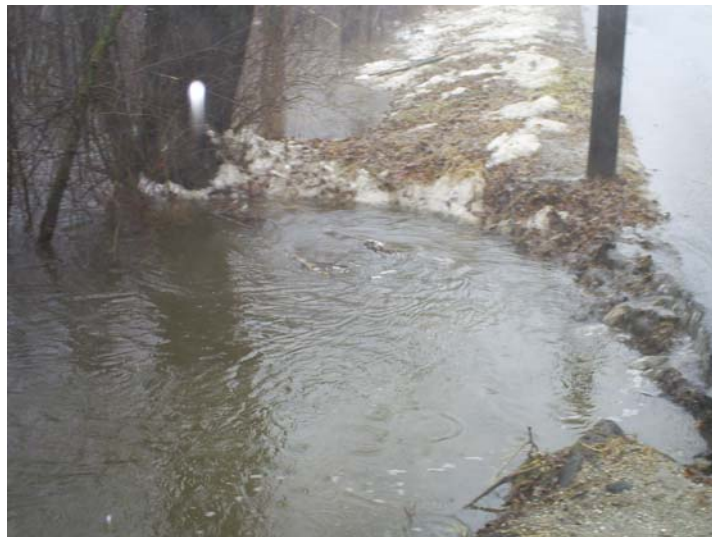
16. An undersized culvert appears stressed due to the substantial precipitation
