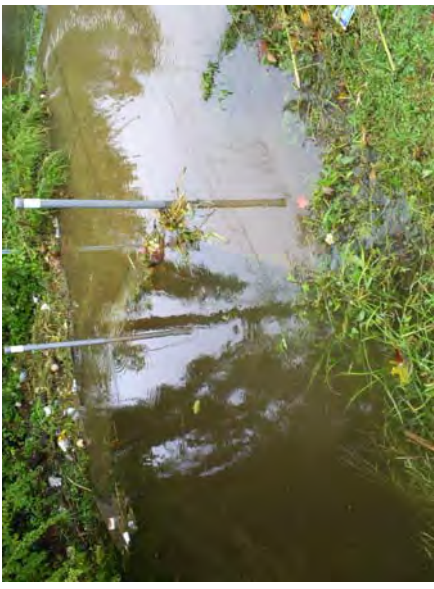
Photo 35: Beginning of Memorial Drive to Overlook Road culvert flooded
