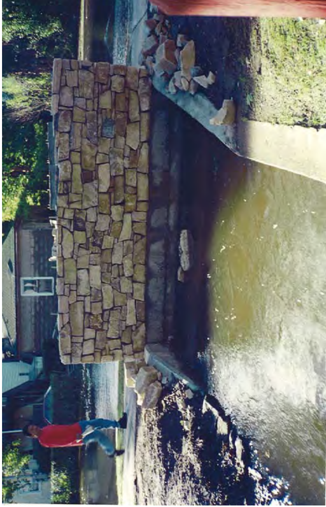
East Pearl Street bridge damage
