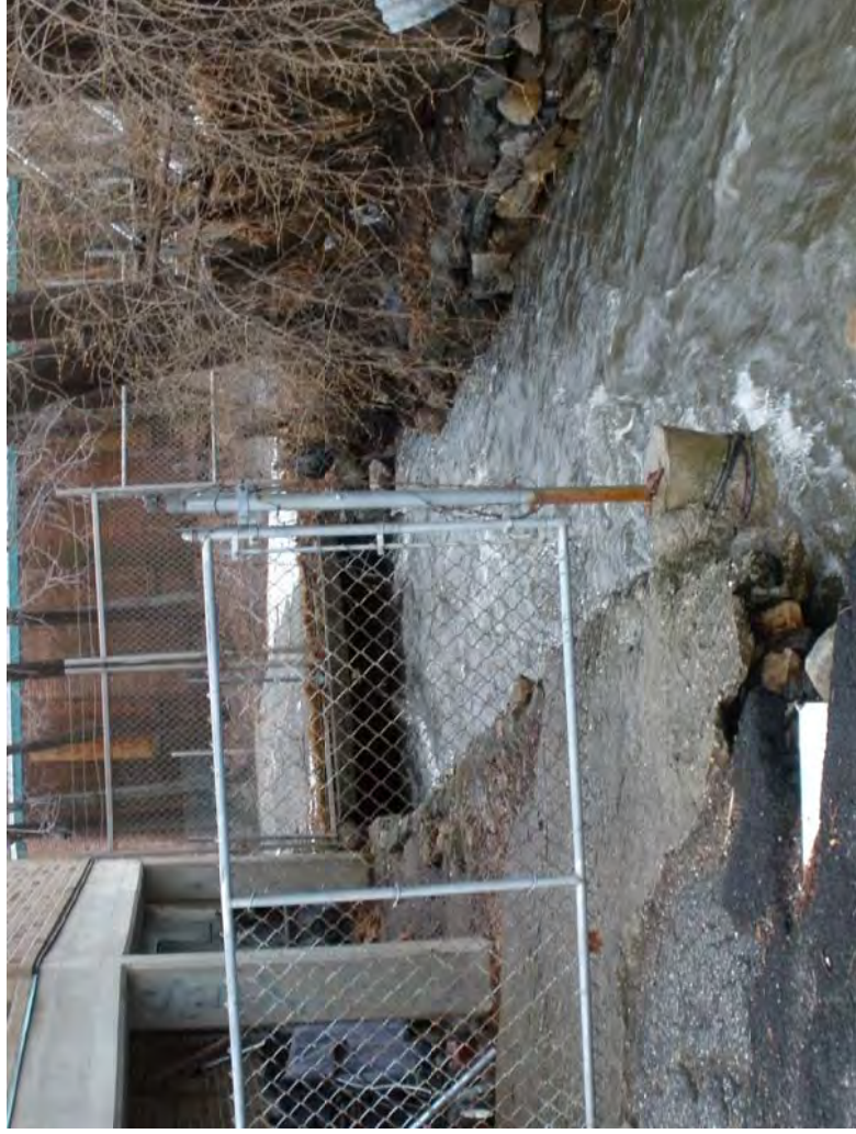
Blind Brook from William Street downstream of George Street, looking downstream at West Street culvert inlet
