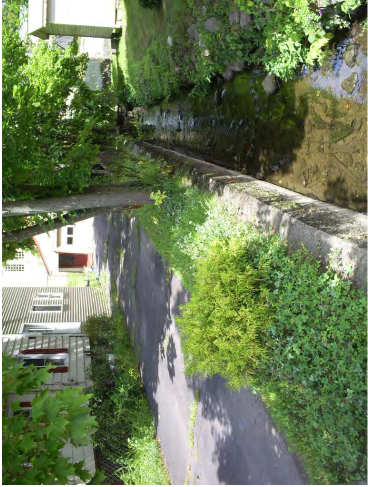
Constricted channel downstream of East Pearl Street bridge over Blind Brook culvert. Repetitive loss property is to left. Note 90-degree turn to right behind shed.
