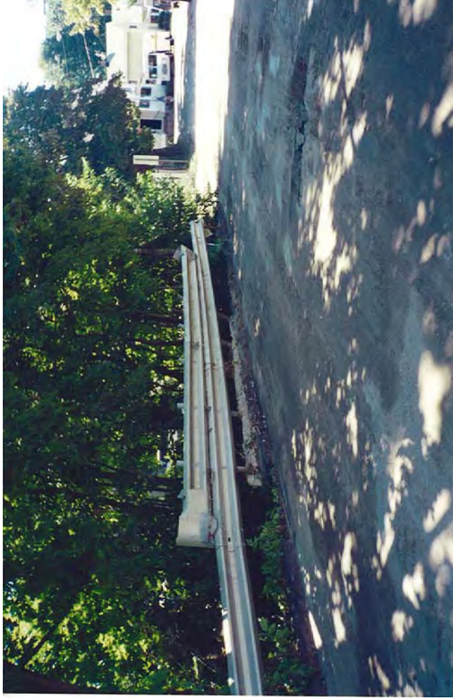
Thorpe Street Extension roadway damage
