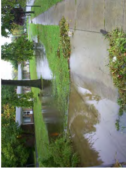
Photo 36: Overflow flooding downstream of culvert
