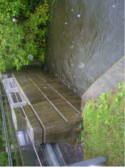
Photo 12: Kissen Brook culvert flooded
