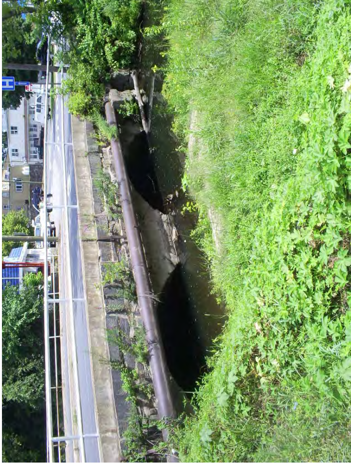
West Avenue bridge over Still River east of railroad tracks, looking downstream from repetitive loss property. Constriction of flow likely exacerbates flooding.
