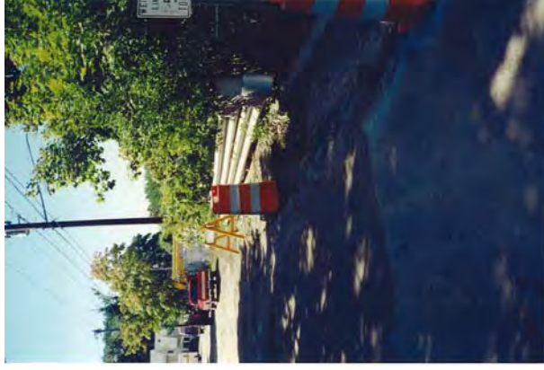
Thorpe Street Extension - Washout
