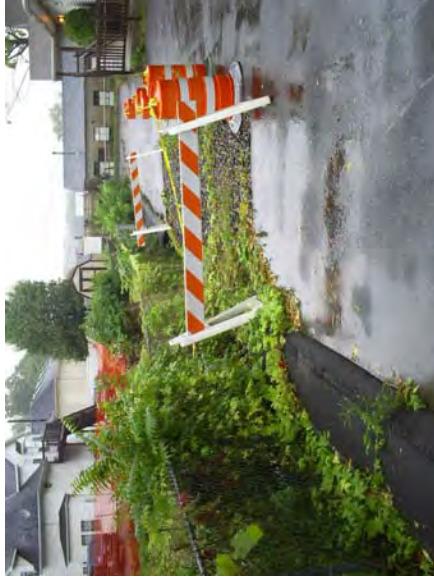
Photo 32: Parking lot undermined at shelter
