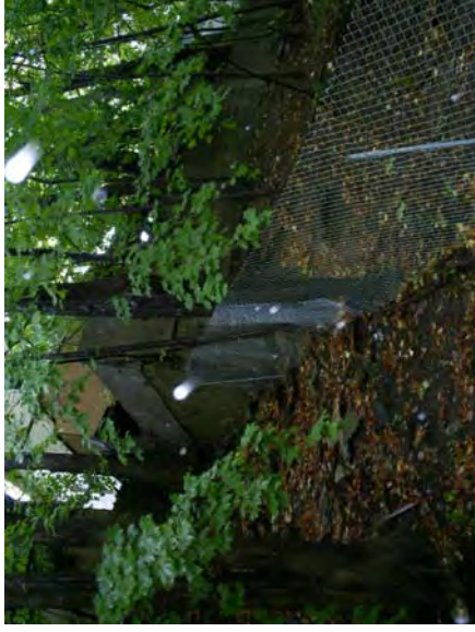
Photo 28: Concrete structure failure above brook
