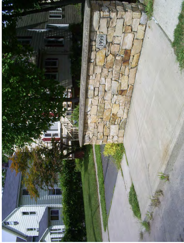
East Pearl Street bridge over Blind Brook culvert, replaced following Tropical Storm Floyd.
