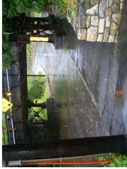
Photo 1: Poor drainage under railroad bridge
