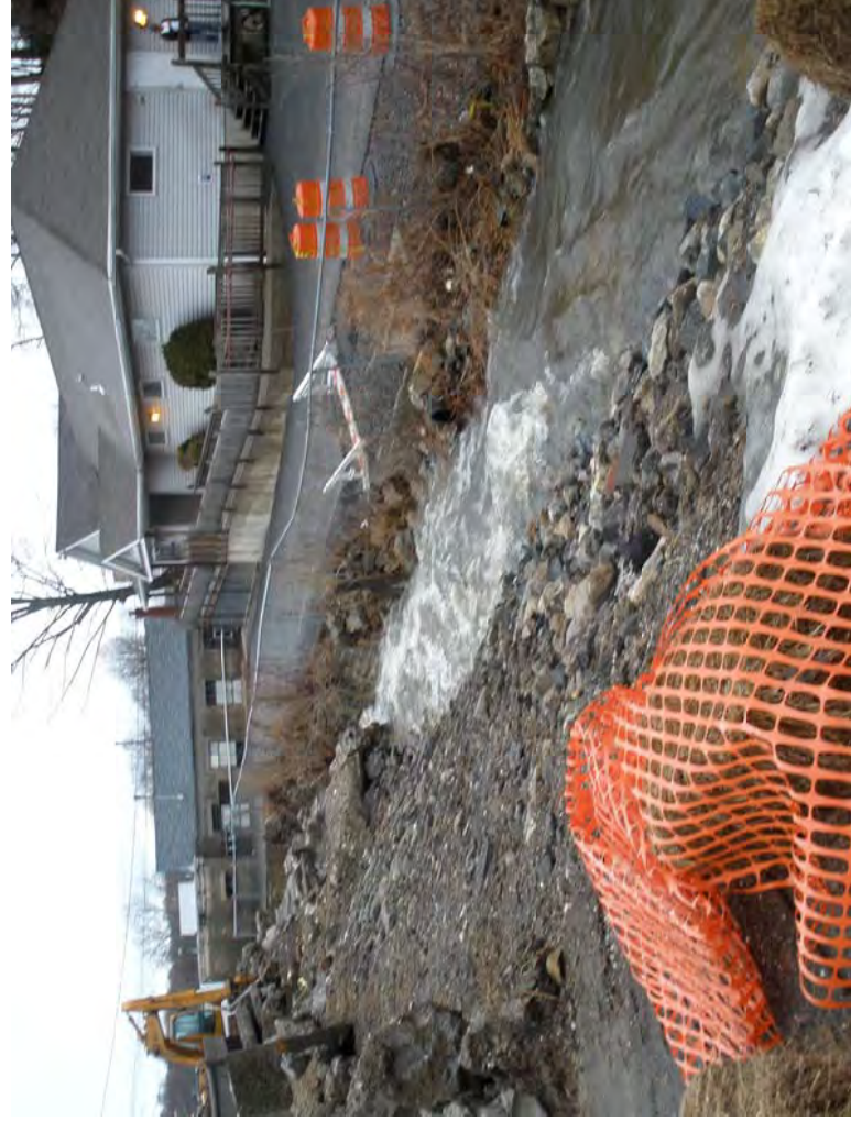
Blind Brook at Pentecostal Church on New Street. Flooding caused major erosion to west bank of stream (church parking lot). Homeless shelter in background.
