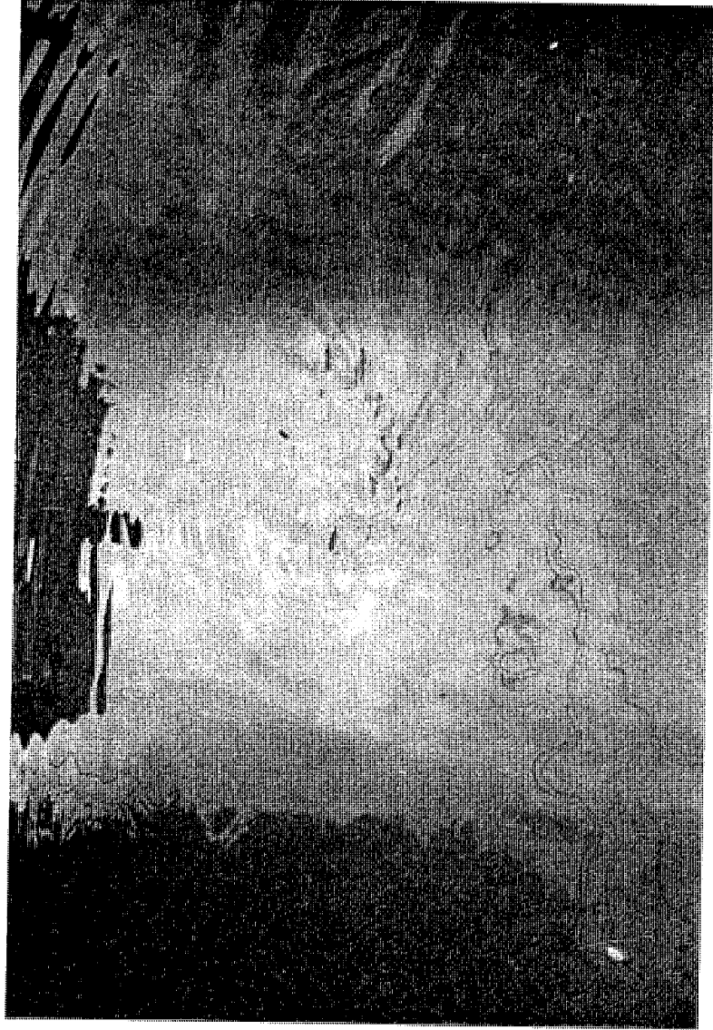
The drains are flowing again and the water is actually going down but everything stinks.
