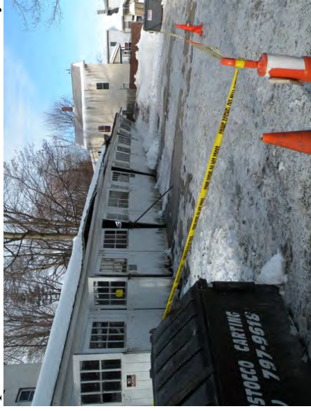
Late January roof collapse of a garage on West Street in Danbury. Photo by Mark Langlois ( http://danbury.patch.com ). Used with permission.
