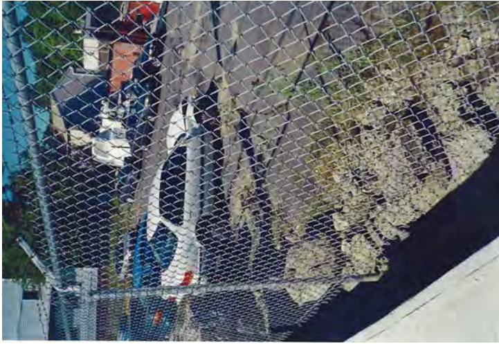
Montgomery Street / New Street. Note damaged car
