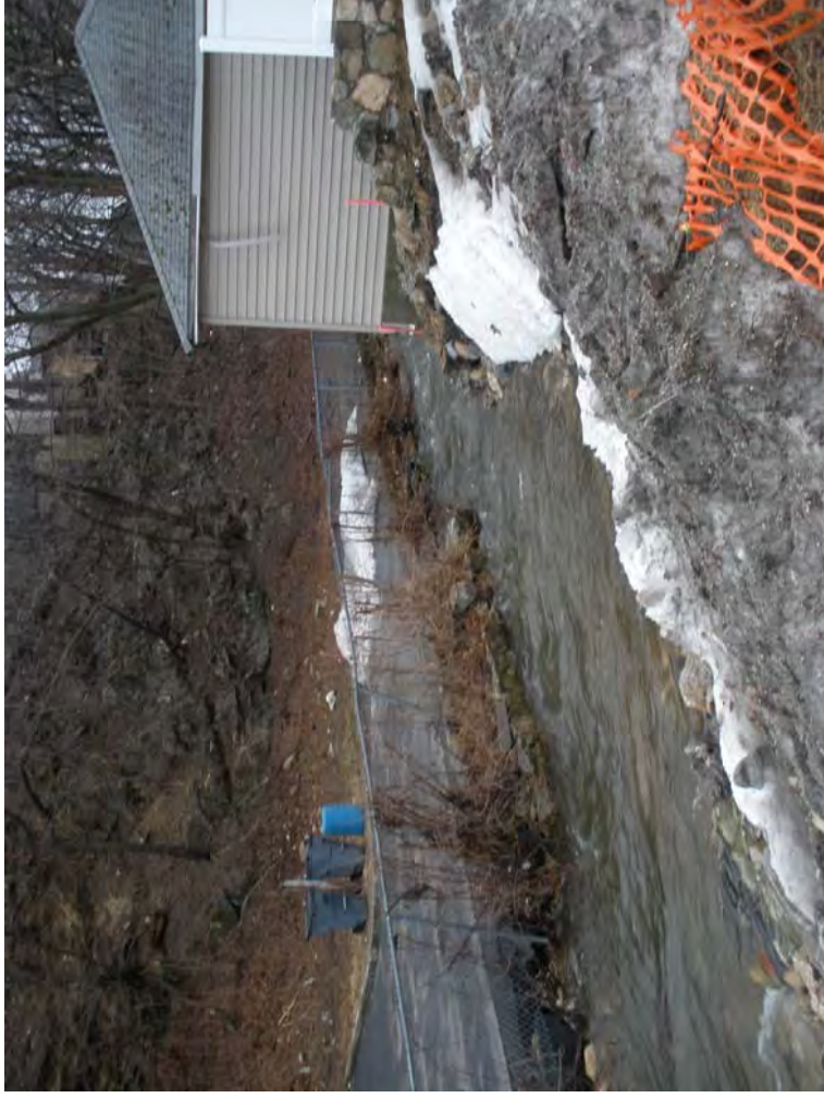
Blind Brook at Pentecostal Church on New Street. Note erosion damage to parking lot in foreground.
