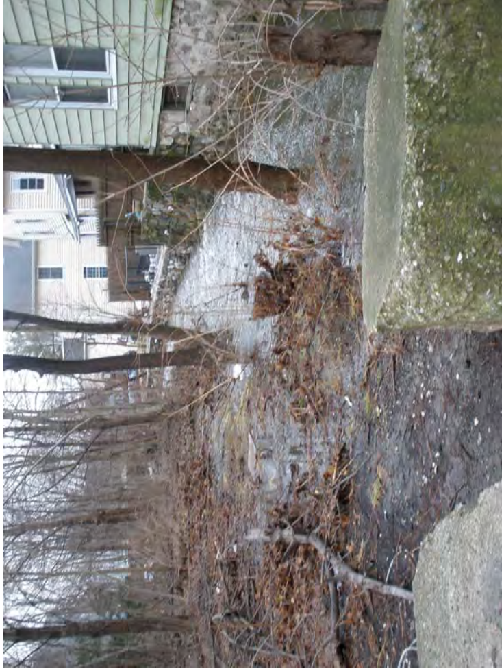
Blind Brook at George Street looking south (upstream). Note culvert wall to right and trees demarking left edge of channel.
