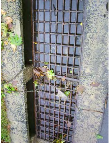
Photo 24: Upstream storm drains full on E. Pearl St.
