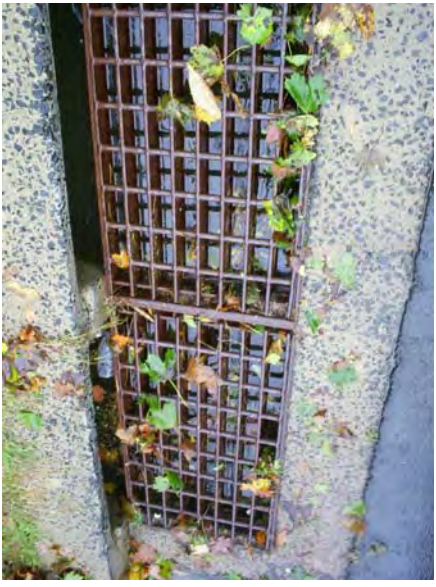
Photo 23: Downstream storm drains full
