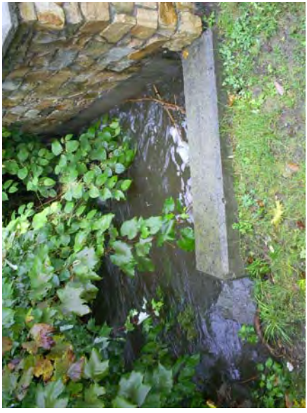
Photo 25: East Pearl St. culvert flooded
