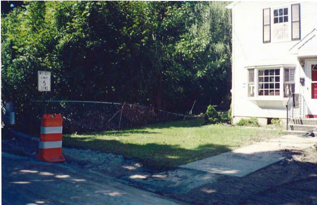
Thorpe Street Extension damaged fence
