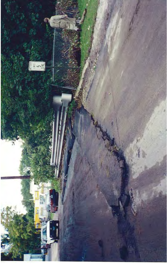
Thorpe Street Extension roadway damage
