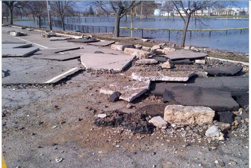
Damage to local infrastructure from Sandy.
