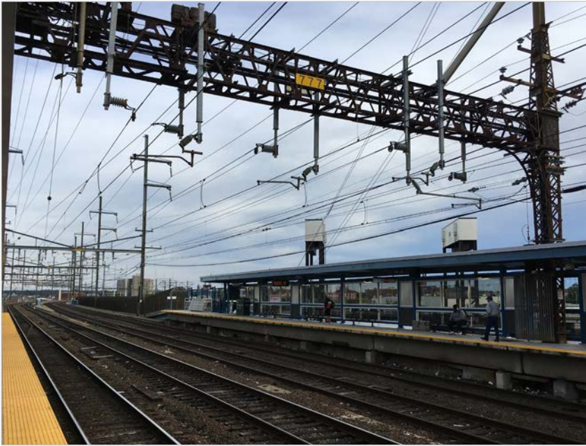
Catenary system in Bridgeport
