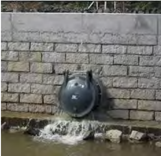
Stormwater Flap Gate
