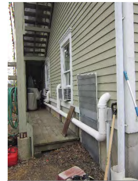
Elevated Pipes 5 Green Hill Place
