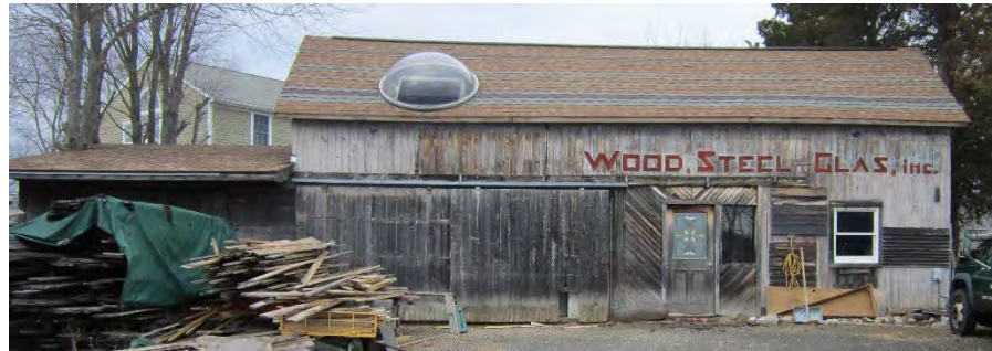
9 Old Post Road Note stains from flooding, opening in sliding garage door, elevated utility to the right.
